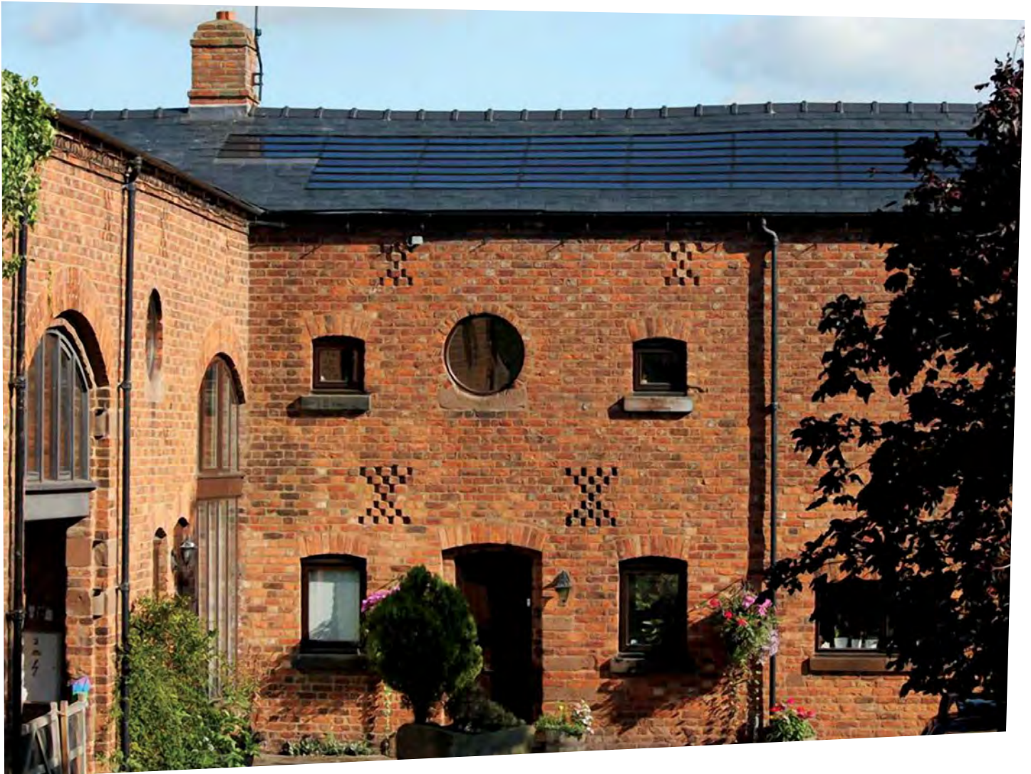
Solar installation and domestic conversion on a listed barn in Chester, installed by The Greener Group.
