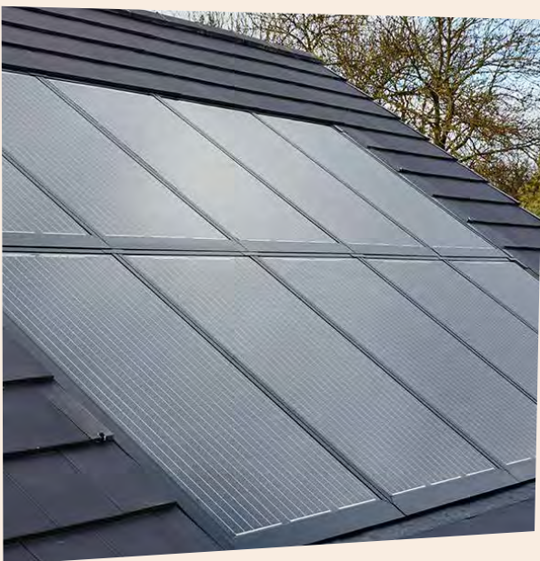
Sunstation: a BIPV solar system that blends into the roof.
