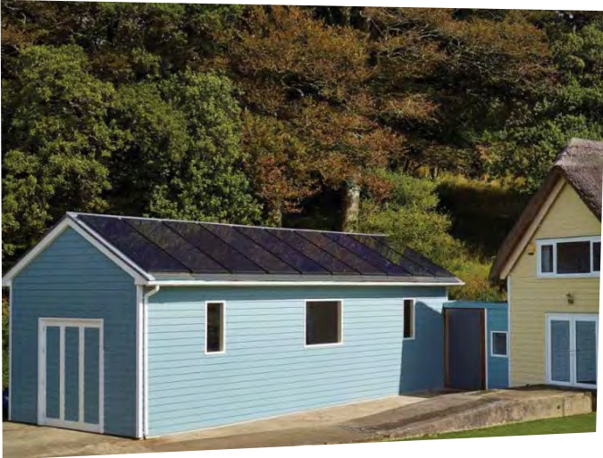
Eight solar panels and two solar thermal panels have been installed on the roof of this building in Cornwall. The panels are identical in size and colour, enabling an effortless combination of different forms of power generation.
