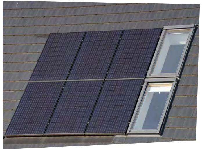
An in-roof BIPV system, designed to complement the roof-light windows.
