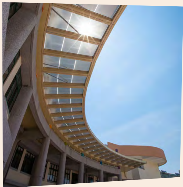
Clear solar glass, a second-generation technology, used as a canopy at a school building, Nantou, Taiwan.
